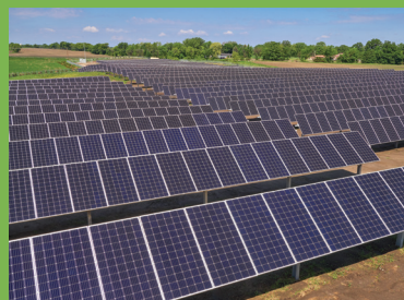
Buffalo Solar 7 MW, Solar
