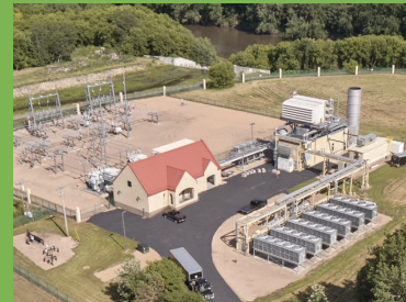
Minnesota River Station 49 MW, Natural Gas
